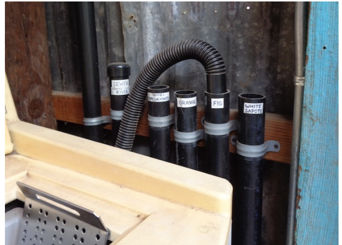
A washing machine discharges graywater to a different pipe with each wash. Each pipe drains to a different edible tree. The soaps used are made for graywater systems.
