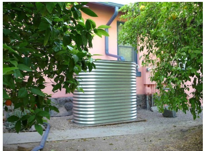
A "slimline" metal tank fits in a narrow space on a small urban lot where it waters adjacent fruit trees and helps moderate temperature extremes.
