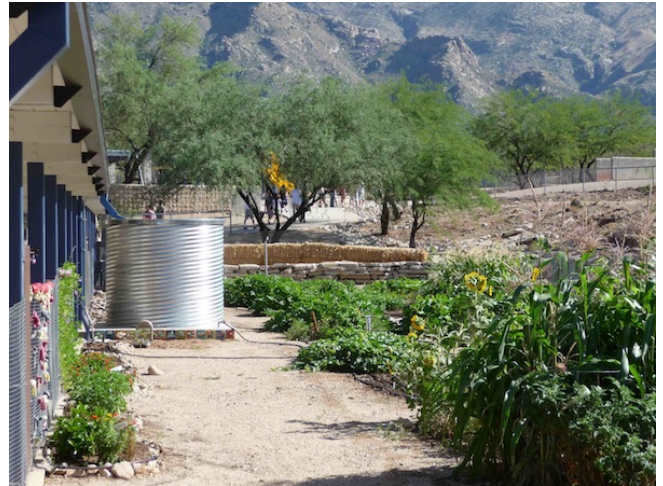
A large galvanized steel rainwater tank is filled from a porch roof and waters the adjacent garden using gravity flow. Since tank elevation is too low to gravity feed water to higher elevation trees, a pump could be added to create sufficient pressure to water higher elevation plants.
